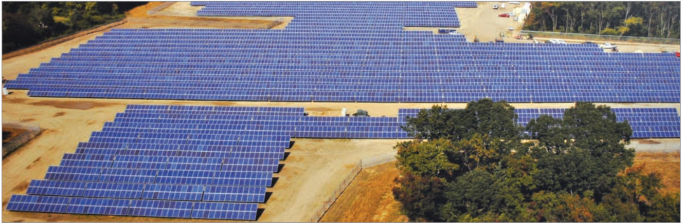
The 2.5 MW Vineland Solar III project, in New Jersey, was completed in November 2011. It is part of a larger, 6.5 MW solar facility for which Vineland Municipal Electric Utility holds a power purchase agreement.
