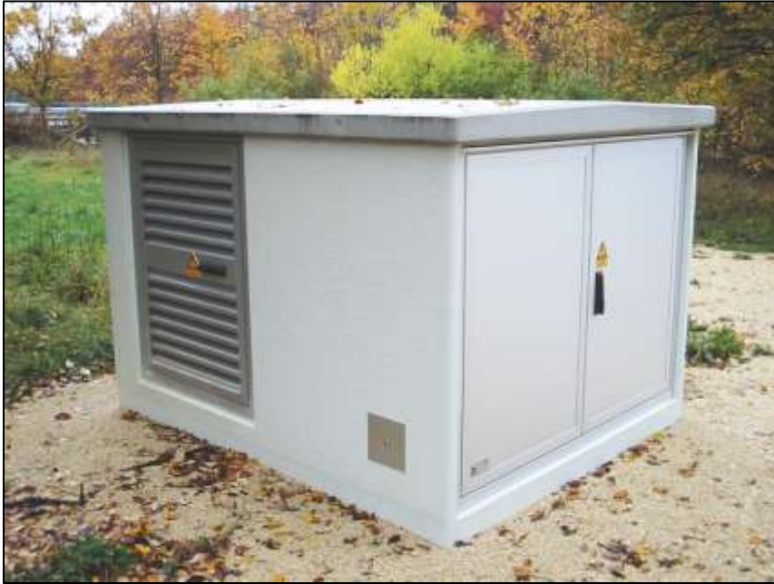
Picture: Typical 20 kV / 400 V transformer station used in Germany
