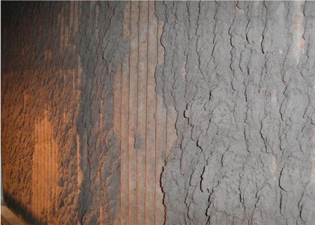
Figure 2. Boiler Tube Fouling ( http://www.intelligent-sootblowing.com/Seiten/slaggingandfouling.html )
