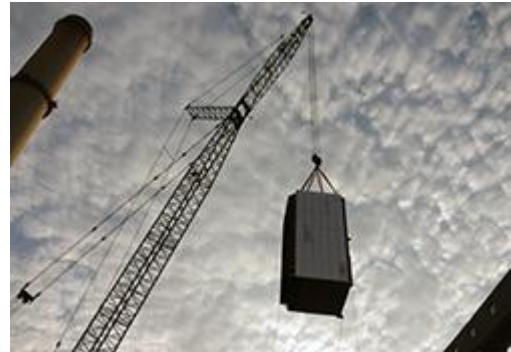
A section of ductwork is lifted into place during construction of the scrubber at the Leland Olds Station.
